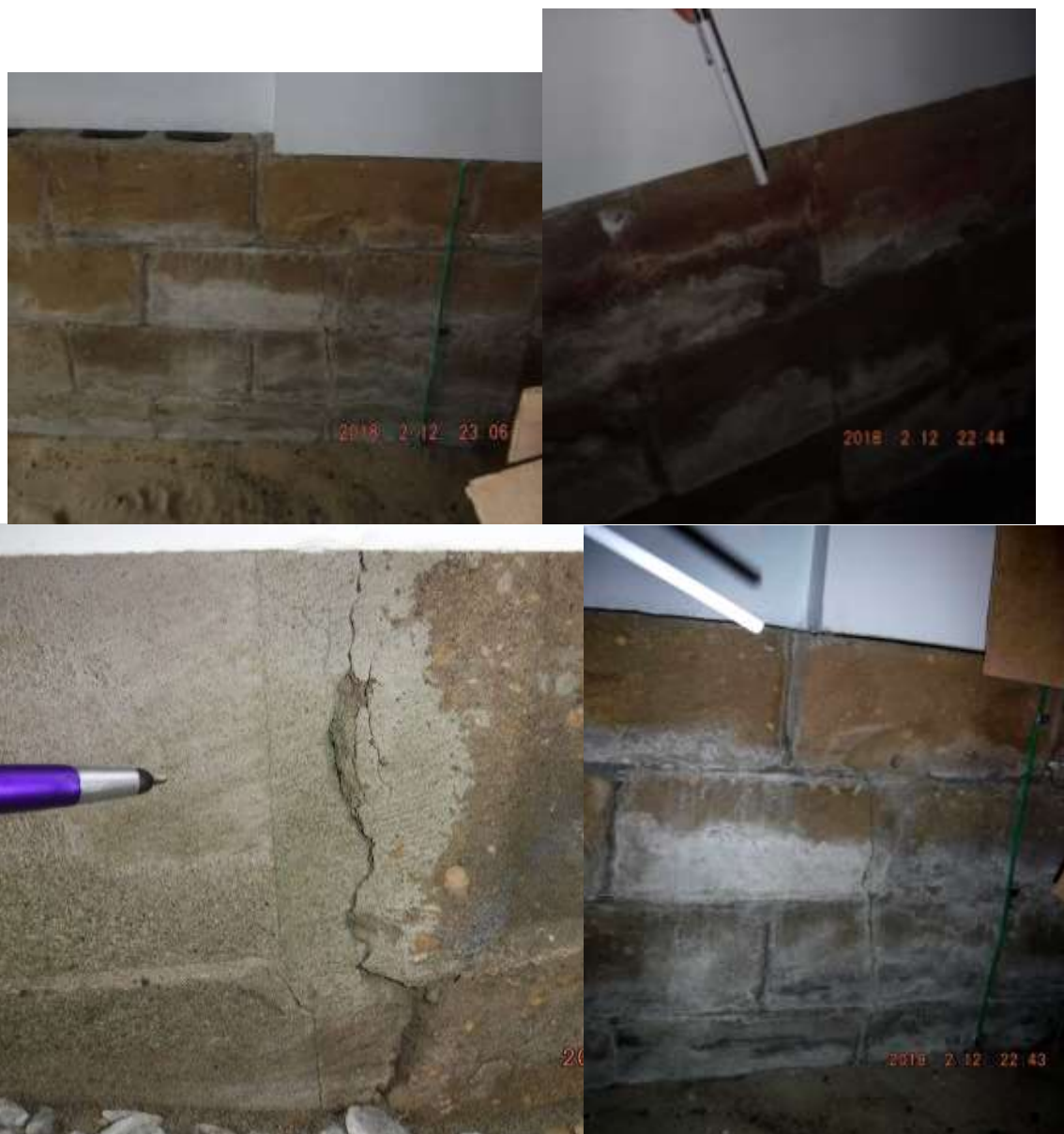
Figure 6 Examples of foundation cracks ( vertical & step) go through the block; visible in garage and exterior. Foundation and sand floor was wet; water seepage into the garage and rear two finished rooms on lower level.
