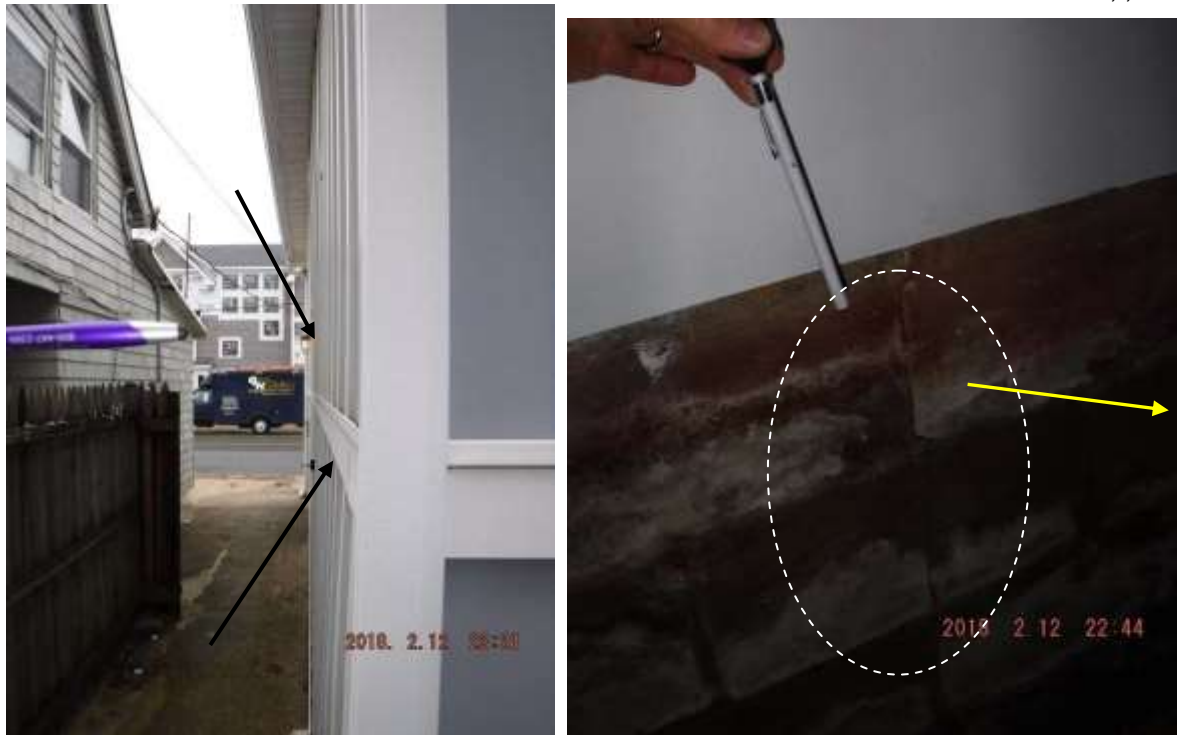
Figure 5 Example of bowed walls as viewed on exterior. The foundation walls in garage had cracks and bowed inward.
