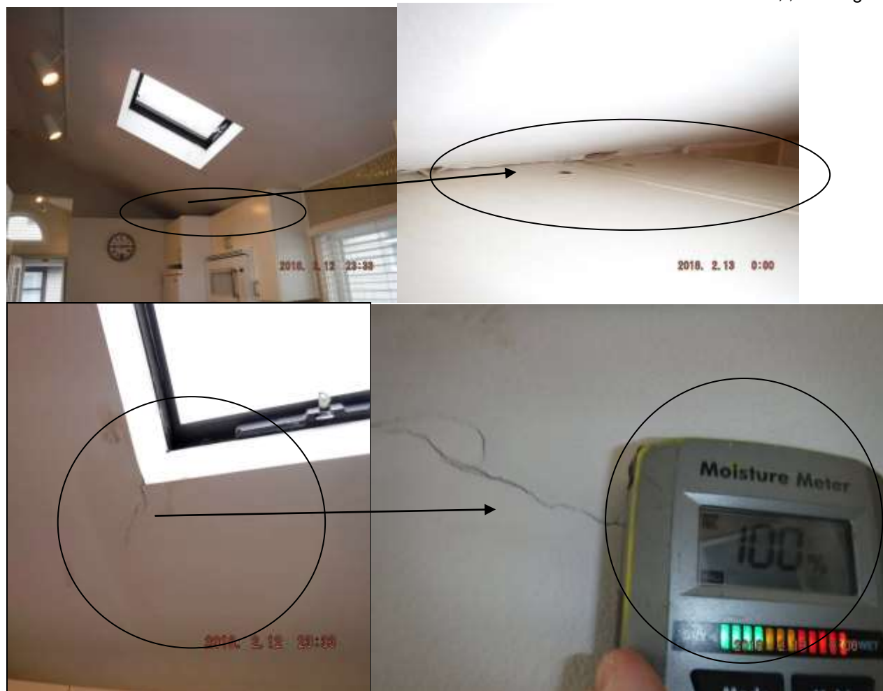
Figure 2 Examples of active leaking (100%) in kitchen; water stains/yellowing and peeled paint on drywall around skylight and above cabinets.
