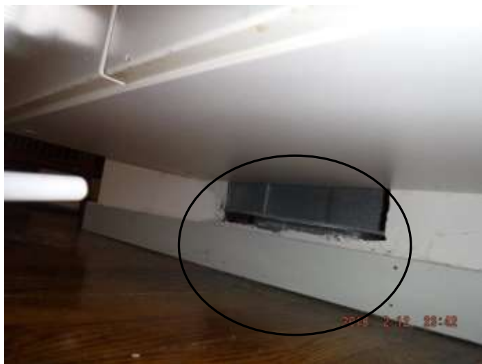
Figure 10 Partially covered HVAC register; improperly installed cabinet. Have an HVAC contractor and/or building contractor evaluate and advise on vent relocation or cabinet relocation.
