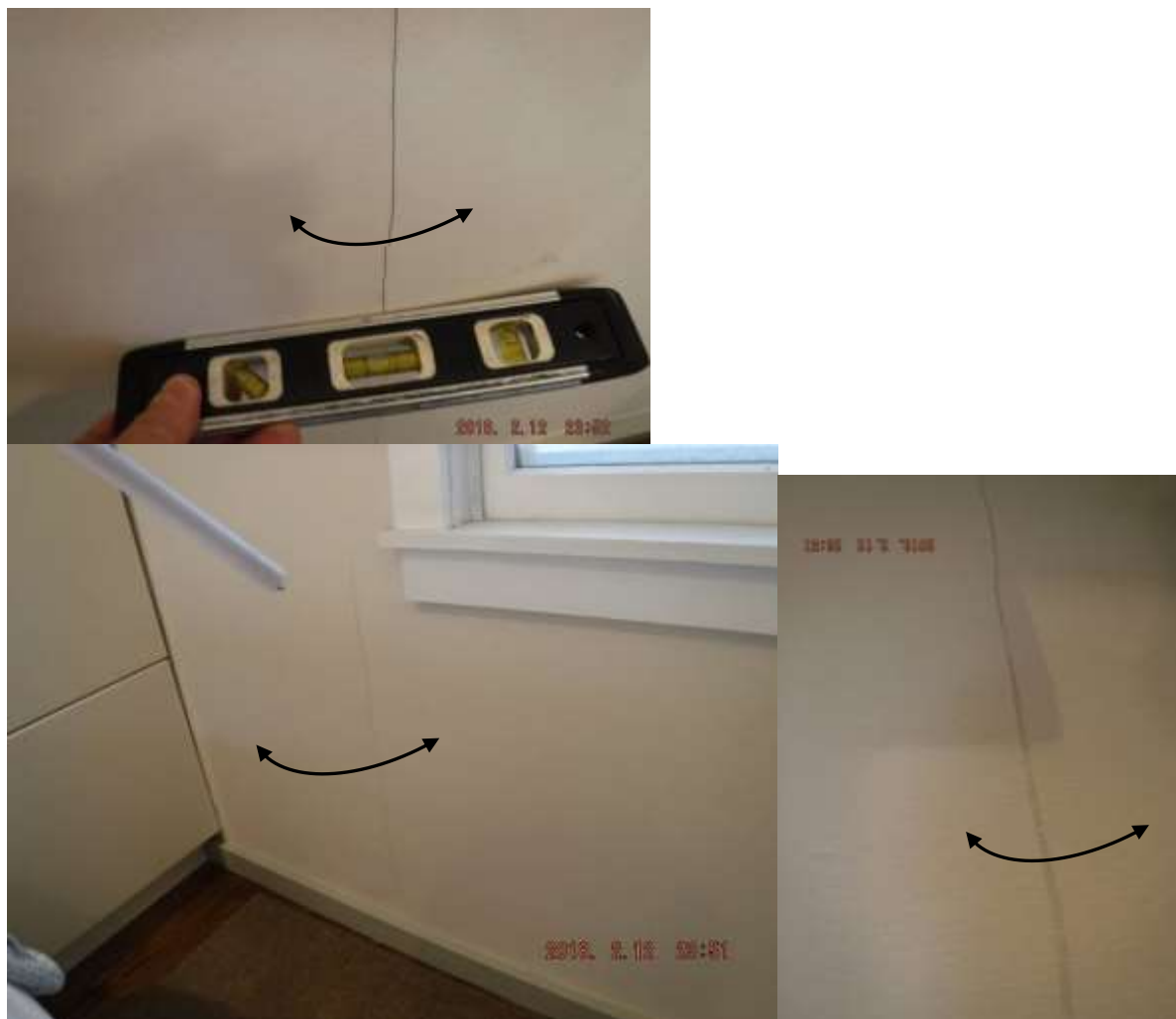
Figure 12 The level rocked when placed on wall; not flat or plumb. Wall had cracks and bowed; see structural comments pg. 2.
