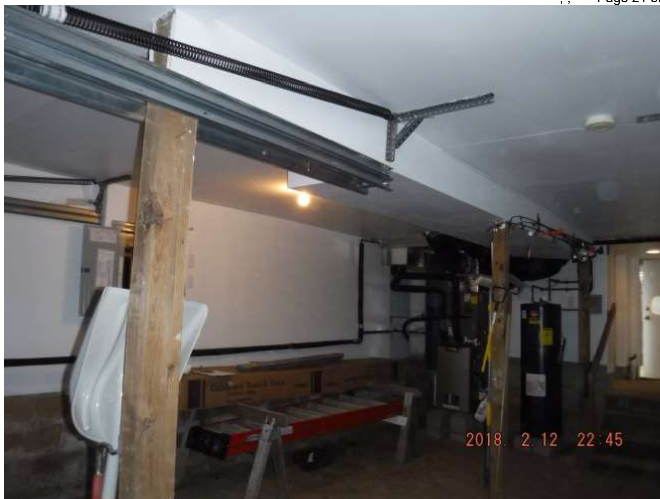
Figure 7 The wood 4x4" posts were undersized and not spaced properly. There were sloped floors in the home above and bowed walls & foundation. See structural comments pg.2. Recommend adding bollards in front of the furnace and water heater for safety.
