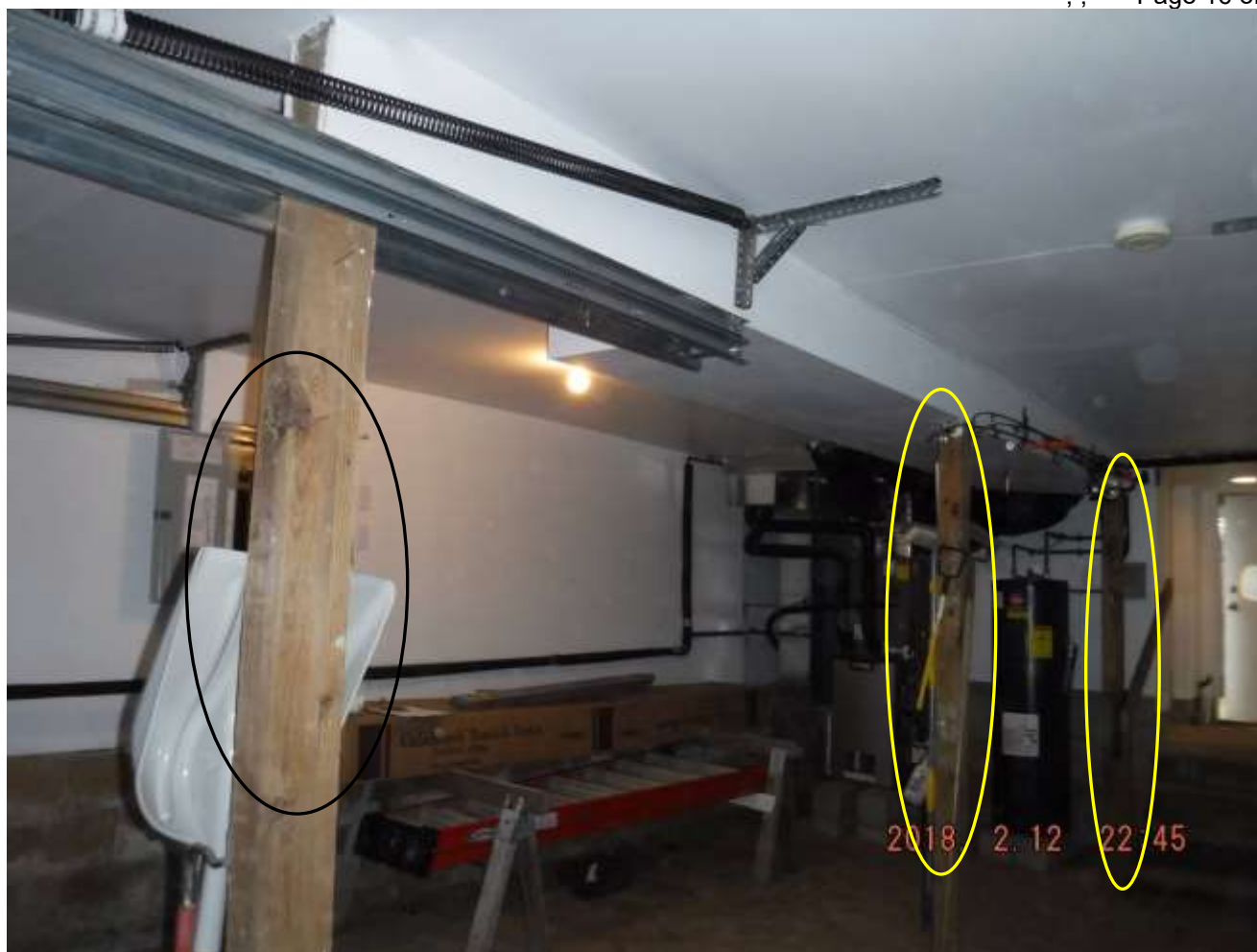
Figure 3 The 4x4" wood columns; under sized and not spaced properly; sloped flooring above in finished main rooms.
