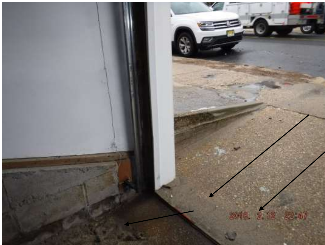
Figure 1 Water entering the garage, wet foundation walls, wet sand floor and musty mold like odor in garage and rear finished rooms.
