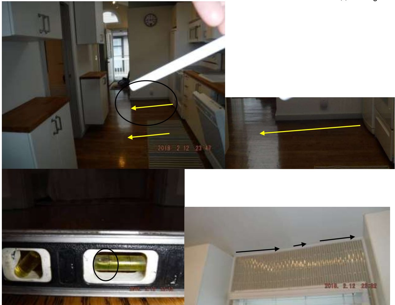
Figure 9 Example of sloped flooring and wavy or bowed walls throughout the home; structural concerns/defects.
