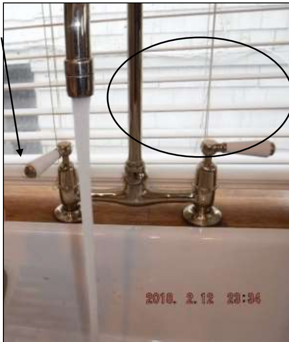
Figure 8 Window blocked by the counter top; unconventional/improper. Recommend a building contractor evaluate and advise. Windows should not be blocked.
